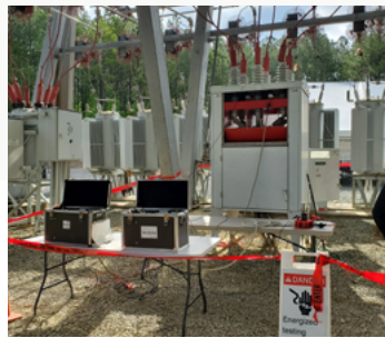
Switchgear and Circuit Breakers
