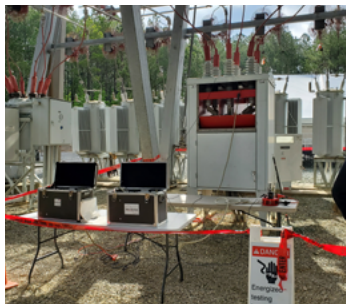
Switchgear and Circuit Breakers
