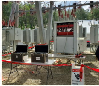
Switchgear and Circuit Breakers
