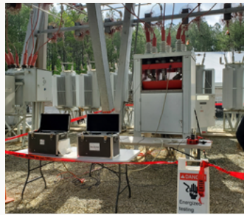
Switchgear and Circuit Breakers
